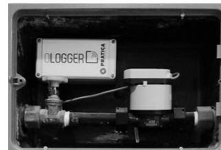
Figure 7. Household flow meter with datalogger deployed
